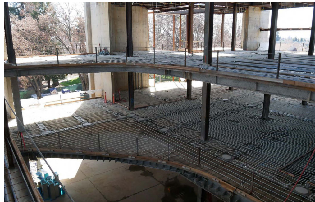
Radiant Heated/Cooled Floors & Infloor Electrical/Data Services
