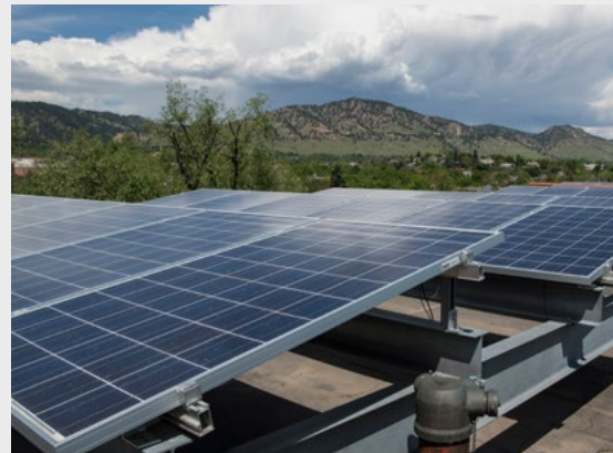
A tilted-rack mounted rooftop solar PV system.
