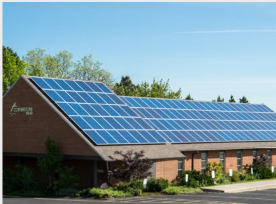
A flush-mounted rooftop solar PV system.
