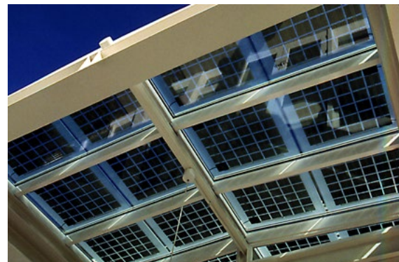
Skylighted entryway featuring solar PV laminated to glazing provides electricity as well as shade and daylight.
