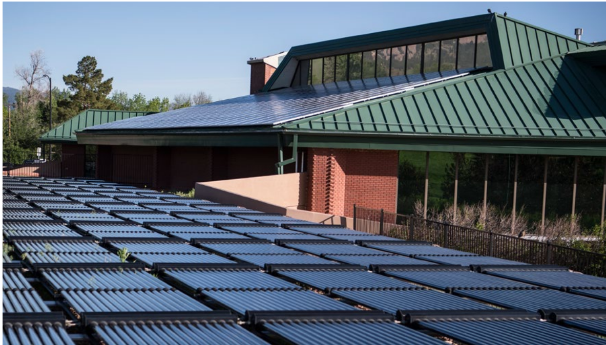
This recreation center features an active solar thermal system using evacuated tube collectors (foreground) that provides heat for a large public swimming pool. The solar PV on the roof provides electricity.
