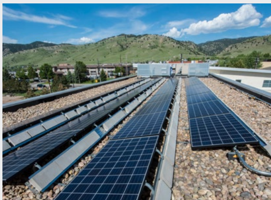
A rooftop solar PV system with ballasted footing mounts.
