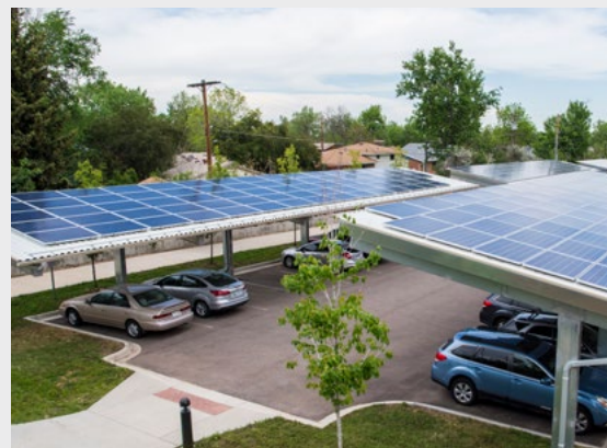
Solar PV flush-mounted to a carport/shading structure.
