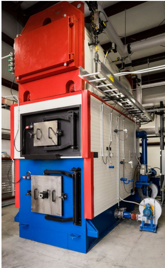
A community/very small bioenergy-fueled district system (4–6 block radius) in Burns, Oregon. The system provides hot water heat to the county circuit court, sheriff's office, and jail as well as an elementary school and a mental health center. The new one-boiler system replaced three oil boilers. Because modern equipment is more efficient, it uses less resource to achieve desired heat and/or power output and has less impact on air quality.
