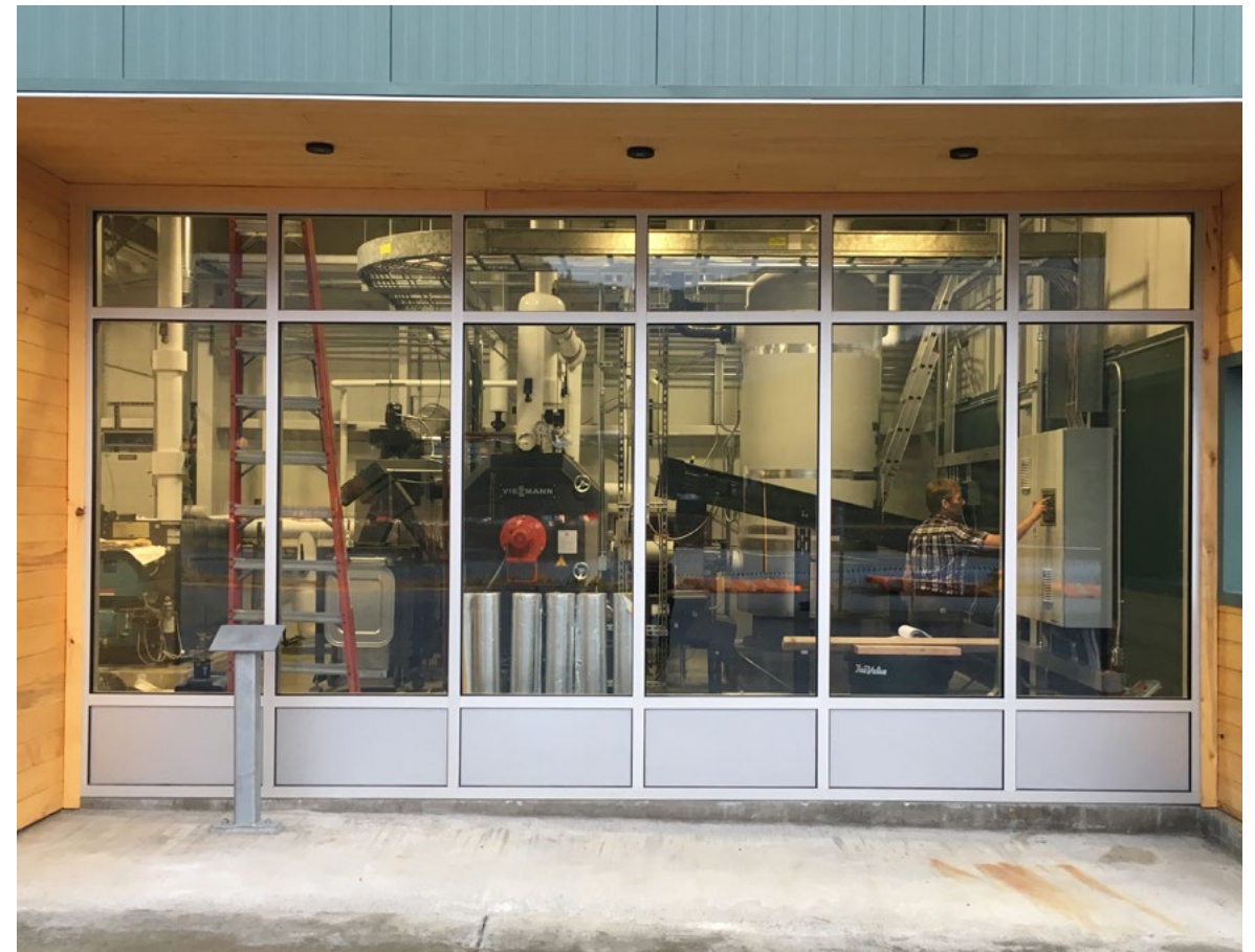
A pellet-fueled boiler system in the Ketchikan, Alaska, airport. Current generation bioenergy equipment benefits from decades of R&D and is currently cleaner, more efficient, and smaller than its predecessors.
