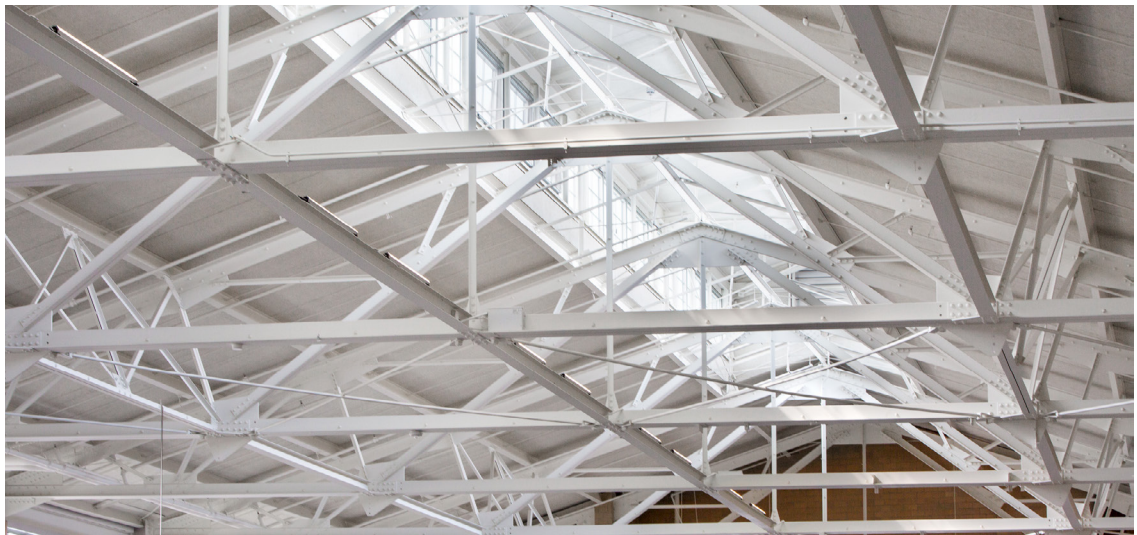
Figure 9: Employees love working in the space, which is filled with natural light even when it's overcast thanks to two roof monitors that run the length of the building. Ortlieb's Bottling House. Image credit: Michael Moran/OTTO
