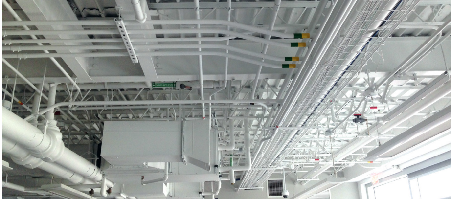
Figure 4: from one another and from the envelope of the building helps ensure that the building's mechanical, electrical, plumbing, IT, and other services can be maintained, replaced, or upgraded without damage to the building or to other services. Image credit: Brad Guy, AIA
