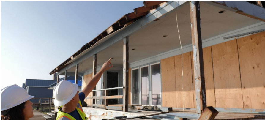
ABOVE: Architects perform building safety assessments after Hurricane Harvey. Source: The American Institute of Architects
