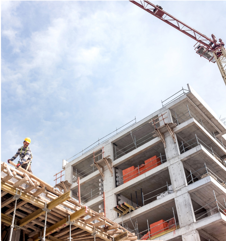
ABOVE: NRMCA advocated for, and helped pass into law, a bill allowing an insurance rebate for compliance to the IBHS Fortified program for commercial construction. Image credit: NRMCA Build With Strength
