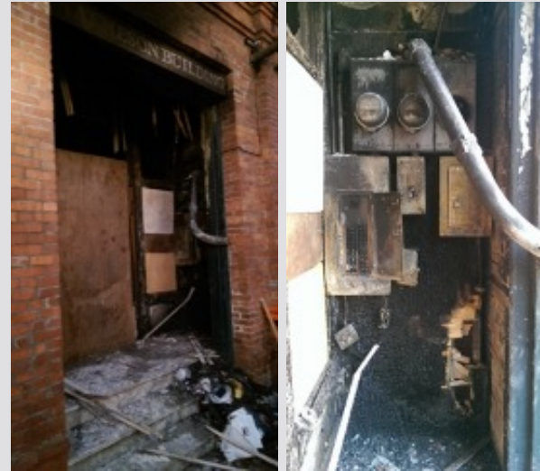
Electrical panel post-fire
